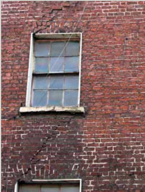
Façade brickwork showing evidence of structural movement in the cracks stretching between the windows
