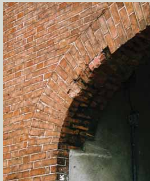
Bricks can be damaged by impact, in this case from a vehicle striking a brick archway
