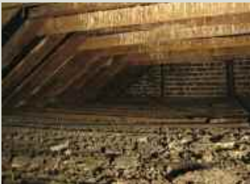
Undersized, long-spanning ceiling joists in this late eighteenth-century roof have become overloaded with pieces of fallen parging and pigeon guano, leading to deflection of the joists
