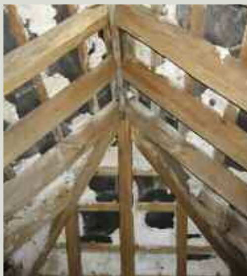
Remnants of parging to the underside of slates
