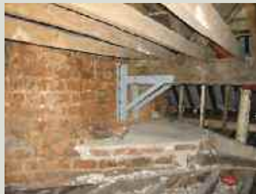
A new steel support bracket has been supplied to support this roof beam severely affected by wet rot at a chimney breast. The chimney flashings above, which had failed, were also repaired as part of these works
