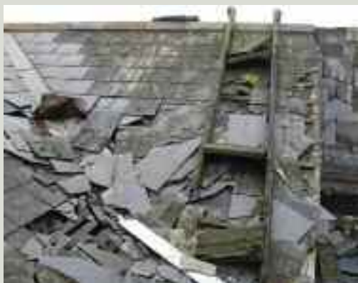
The theft of lead and copper from a historic roof can cause significant damage and leaves the interior of the building vulnerable to further damage from flooding
