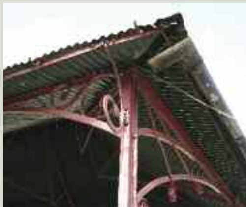
This corrugated iron is suffering from pitting, visible as small pinpricks of light where the metal has corroded through. There is also crevice corrosion occurring at the junction of the sheet with the hip roll. In addition, work is urgently needed to repair the rainwater goods
