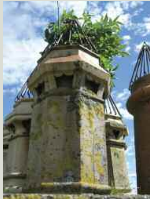
The use of wire crown guards prevents birds from nesting in chimney pots, but does not stop plants rooting in blocked flues
