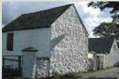
The flush verge detail, as seen in this example, is vulnerable to the extremes of weather; the reconstruction of the detail using lime mortar is of particular importance to ensure that there is sufficient tolerance and flexibility for the slates to move
