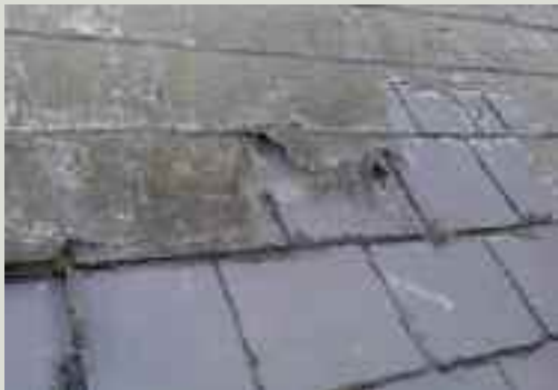
The process of covering a leaking slate roof with a bitumen covering was known as 'turnerising.' It is ineffectual and damaging and should never be carried out on a historic roof. Furthermore, it prevents the slates ever being salvaged for reuse
