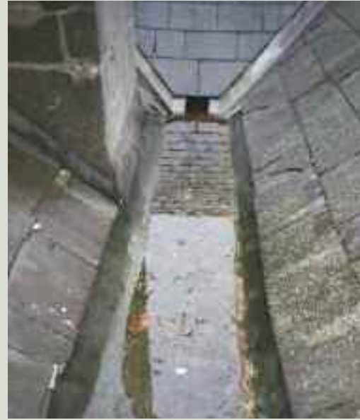
View of a defective valley gutter with a shallow fall that is now holding water. Birds' nests in the outfall of the secret gutter (seen at the top of the image) blocked this roof outlet
