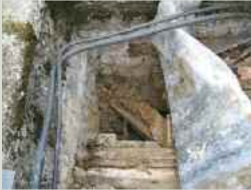
Rot beneath this section of parapet gutter resulted in localised ponding of rainwater, exacerbating the problem and leading to wet rot damage to the truss end. Note that bonding timbers embedded further down the wall may also be affected by such leaks
