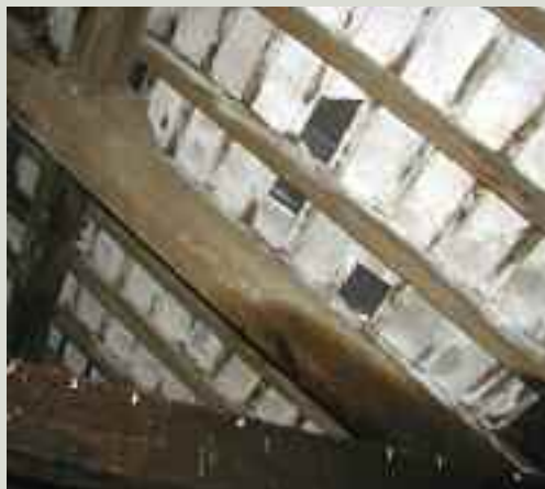
Substantially intact parging to the underside of slates is visible from within the attic space and provides a secondary line of defence against rain and wind entering the interior of the building
