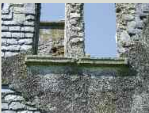
On this ruinous house in County Cork, the vertically hung slates, bedded in lime mortar, were later rendered over. Their existence only came to light as the external render decayed and fell off
