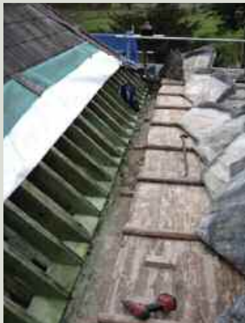
Slight lead corrosion can be seen on the exposed underside of the lifted lead sheeting on the right. The main problem here was a poorly detailed gutter. There was no need to change the regime of the flat roof, although good practice would include an underlay between the deal boards and the sheet lead
