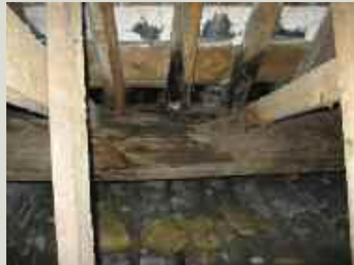
Evidence of wet rot damage to a roof beam and rafters under a tapered valley gutter. Only about ten per cent of the beam section was degraded, so no strengthening works were required to the beam. The rotted rafter ends, however, needed replacement
