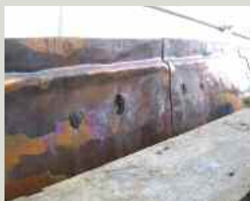
This copper parapet gutter lining has been lifted for inspection following water penetration problems. The bright salmon-coloured areas indicate that corrosion is occurring. Holes in the copper had been previously filled with a bitumen product in an earlier repair attempt which has exacerbated the problem, as bitumen corrodes copper
