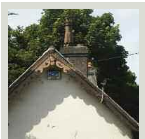
The poor condition of overhanging verges can lead to deterioration of the ends of the purlins as well as the loss of sections of decorative timber bargeboards
