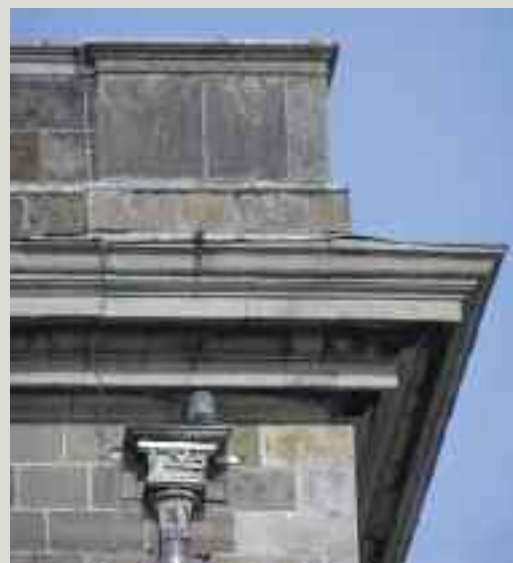
A rare example of a surviving lead hopper head with an embossed date of 1725
