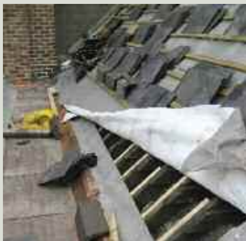
Re-lining a valley gutter in copper. Splice repairs were required to the ends of rafters where the previous valley had leaked over a significant length of time, causing decay of the timber structural elements below
