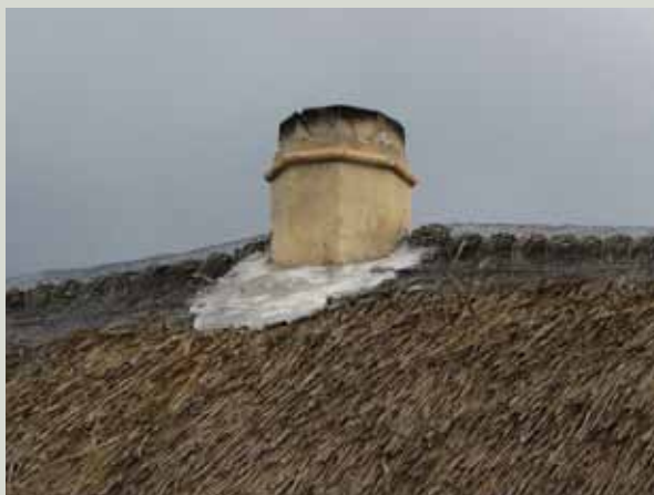
Low-rise chimneys are traditional on thatched buildings. They rely on large chimneybreasts below to ensure that sparks from the fire are extinguished before they reach the upper parts of the chimney
