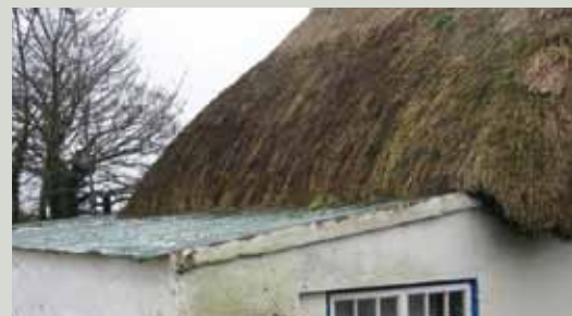
The end of the thatch sits on the lean-to metal roof of an extension. Rainwater shed from the thatch cannot drain properly and will eventually lead to rotting of the thatch
