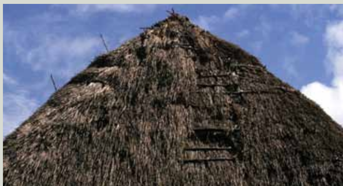
Fixings becoming exposed on the thatch surface indicate that the roof needs re-thatching
