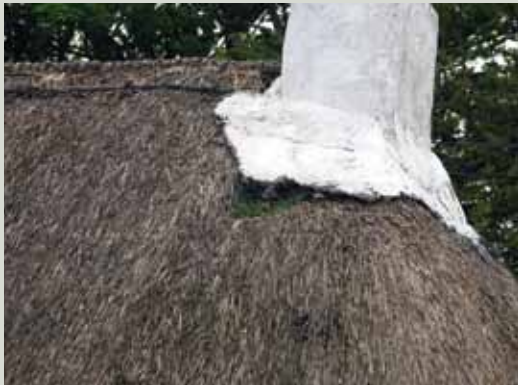
The shrinkage of thatch in vulnerable areas of the roof such as at the base of chimneys facilitates water ingress and should be repaired quickly
