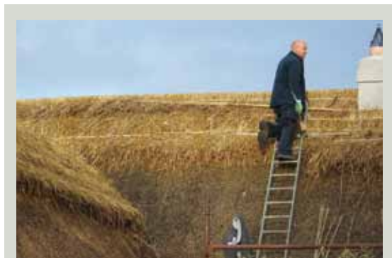
Renewing the ridge of a thatched house in County Meath (Image courtesy of Brian Simpson)
