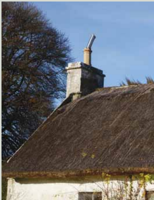
Chimney alterations and flue installations should be carried out by specialist contractors as inappropriate materials and poor workmanship can increase the fire hazard
