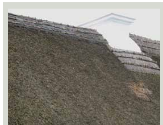
Renewal of vulnerable sections of a roof, particularly the ridge and base of the chimney can extend the lifespan of a thatch
