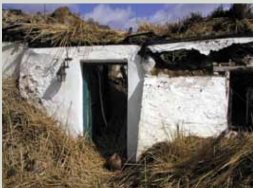
The devastating results of a fire in a thatched building
