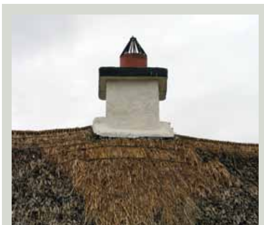
Typical rendered masonry chimney with mortar flaunching at the base and firmly scoloped thatch around it
