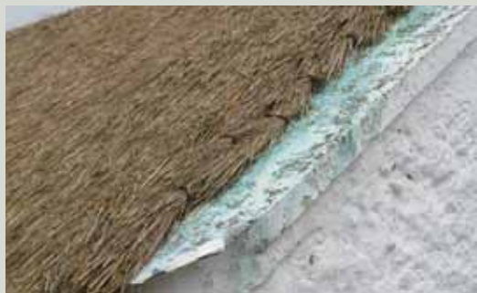
The typical blue run-off of copper sulphate solution can be seen on the verge of this roof indicating that a treatment of bluestone has been applied to the thatch
