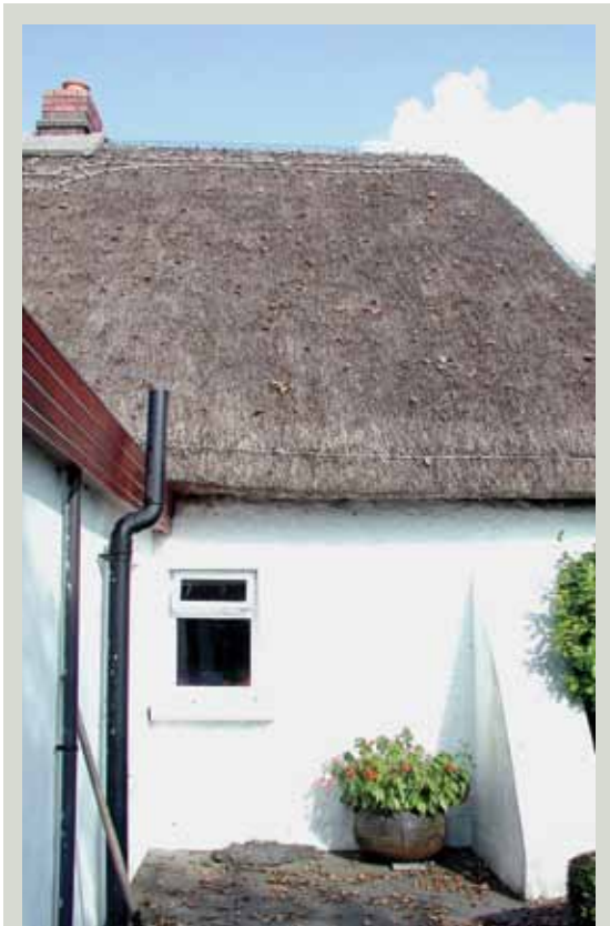
Wire netting can trap fallen leaves, delaying the run-off of rainwater and so accelerating the decay of the thatch
